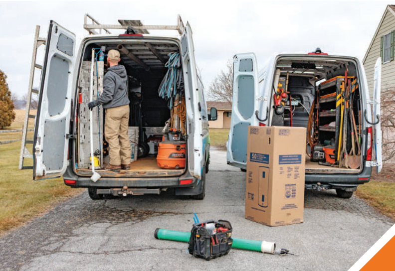
▲ Service Technician James Fink removes supplies needed as a residential job from his truck. The team is installing a new water heater (Rheem) and doing onsite water system maintenance.
